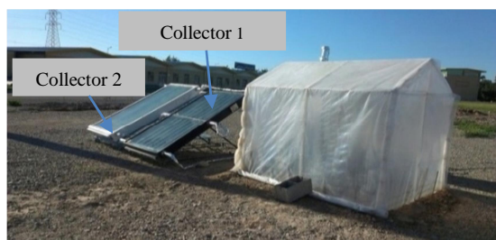
Fig. 2 Real view of greenhouse and heating system
