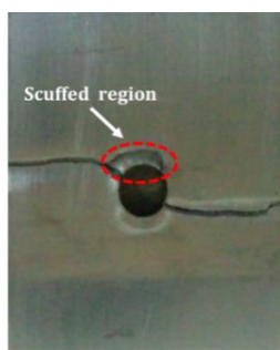
Fig. 10 scuffed region during cyclic loading
