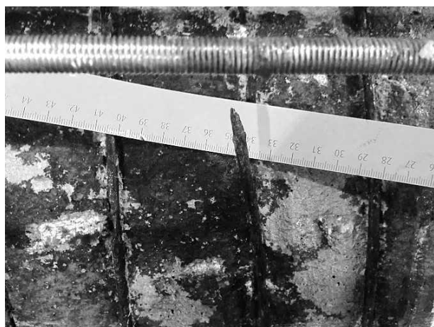
Fig. 23 Corroded state of post-tensioned wires
