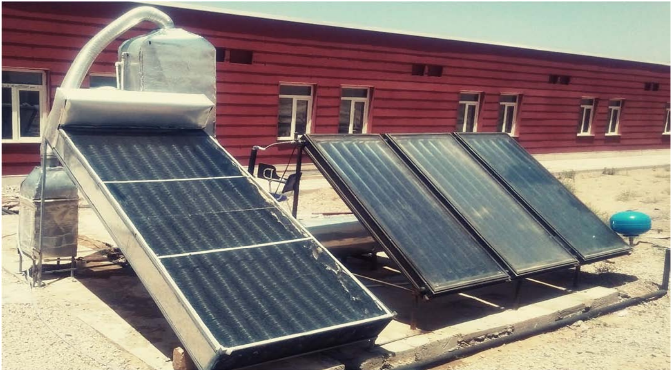
Fig. 2 A view of the manufactured solar humidification-dehumidification desalination system
