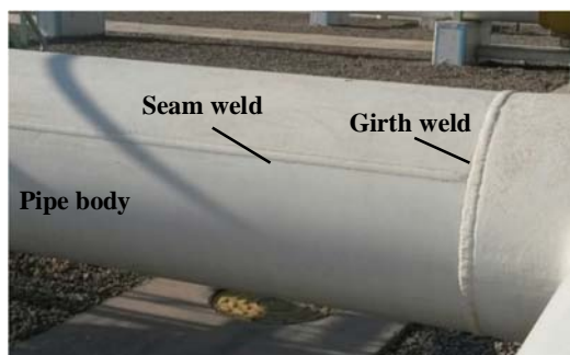
Fig. 1 Photograph of a gas pipeline
