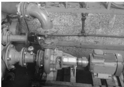
Fig. 3 Test Setup of Centrifugal Pump
